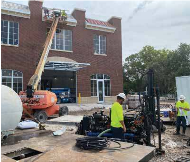
Installers inject dual-component polymers to seal Sarasota Lift Station 87 while construction continues.
