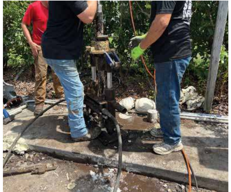
A crew deploys the patented mixing device to 31 feet adjacent to the 10-foot void near the wet well.
