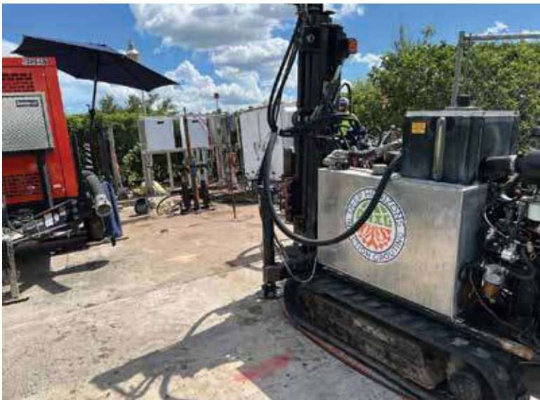
The small equipment footprint allows easy access in tight spaces. The five-day project included four injection points and 2,623 gallons of grout.
