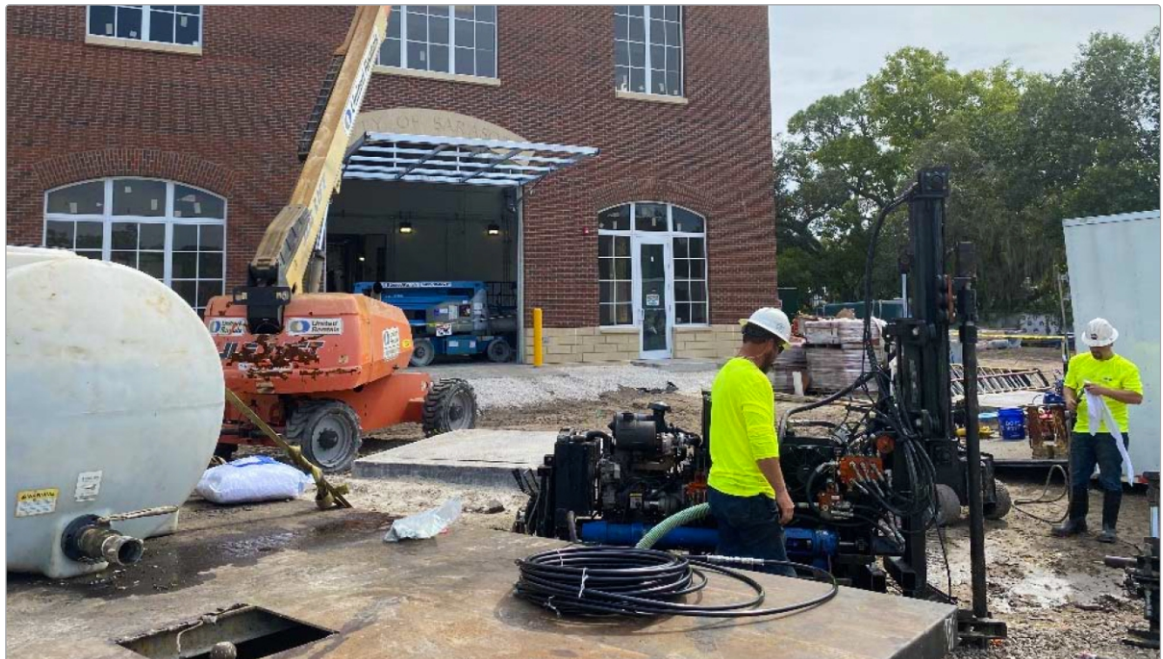
Sealing the buried line while construction continues uninterrupted on the remainder of the lift station infrastructure by the prime contractor.
