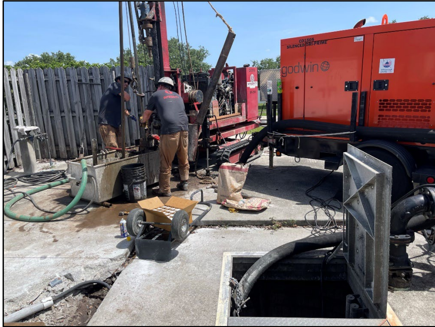
Plate 1 – SPT boring B-1 and Subsided Slab
